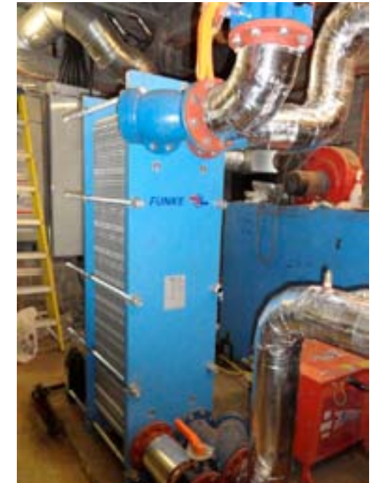
500kW Plate Heat Exchanger in School Plantroom
